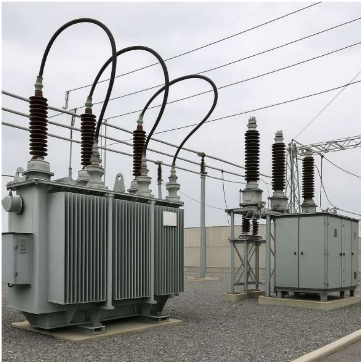
Figure 3. A real-world view of a power distribution substation, showing key components including a power transformer, circuit breakers, busbars, and switchgear.
